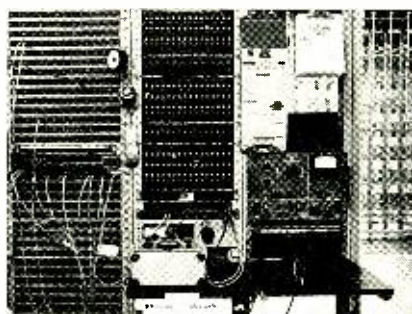
Audio jack-panel and switching board.
